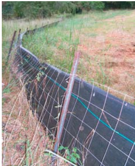
Good installation of "super" (i.e., wire reinforced) silt fence. Note that wire is installed between the fabric and stakes, and provides a web of support as the ponded flow pushes against the fabric. Also, note the grass strip between the bare area and the fence, which helps to slow and filter flows before ponding along the fence line.
