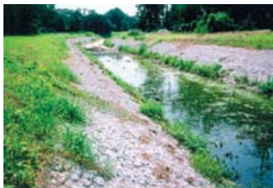
Gabion mattresses can replace turf mats in high-flow, high-velocity channels. Mixing mulch and soil into the rock can help support vegetation for a "greener" look.
