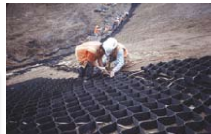
Plastic cellular blanket installed on a steep, long slope. Work closely with manufacturers on these applications to ensure proper design, installation, and initial maintenance.
