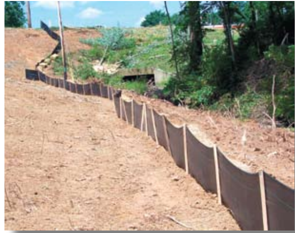
Silt fence installed backwards—note that stakes are on the uphill, rather than downhill, side of the fabric. Ponding flows against this fence will push the fabric away from the stakes, causing failure and releasing sediment to the small stream on the right.
