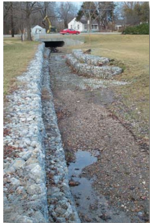
Gabions can protect banks in areas of high velocity flows. Some designers prefer TRMs in these situations, if space is available to slope banks back appropriately.
